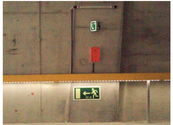
Direction display for emergency escape route
